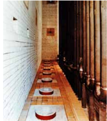
Inside view of a ethylene cracking unit with burners and penetrations
